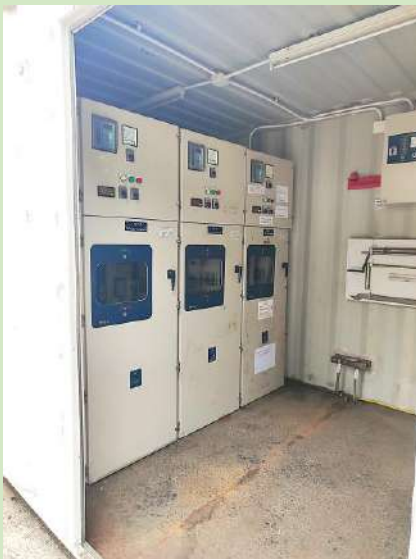
12KV SWITCHGEAR (800A)
