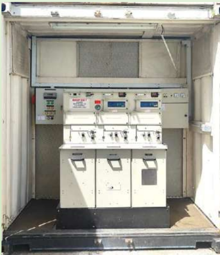
RING MAIN UNIT (RMU) & BATTERY CHARGER
