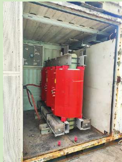
CAST RESIN TRANSFORMER 2000KVA
