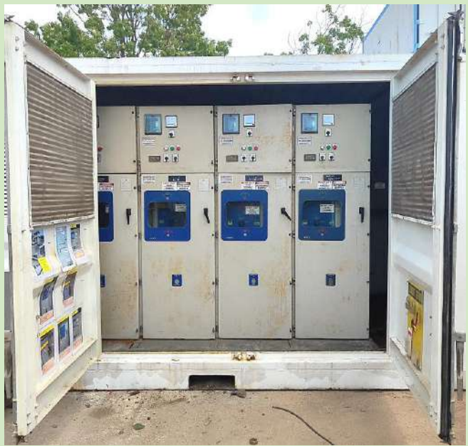
12KV SWITCHGEAR (800A)
