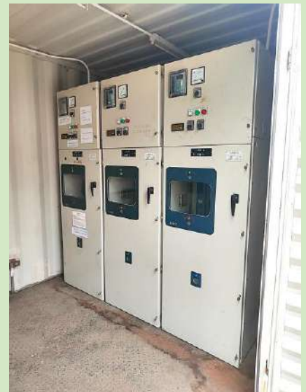
12KV SWITCHGEAR (800A)
